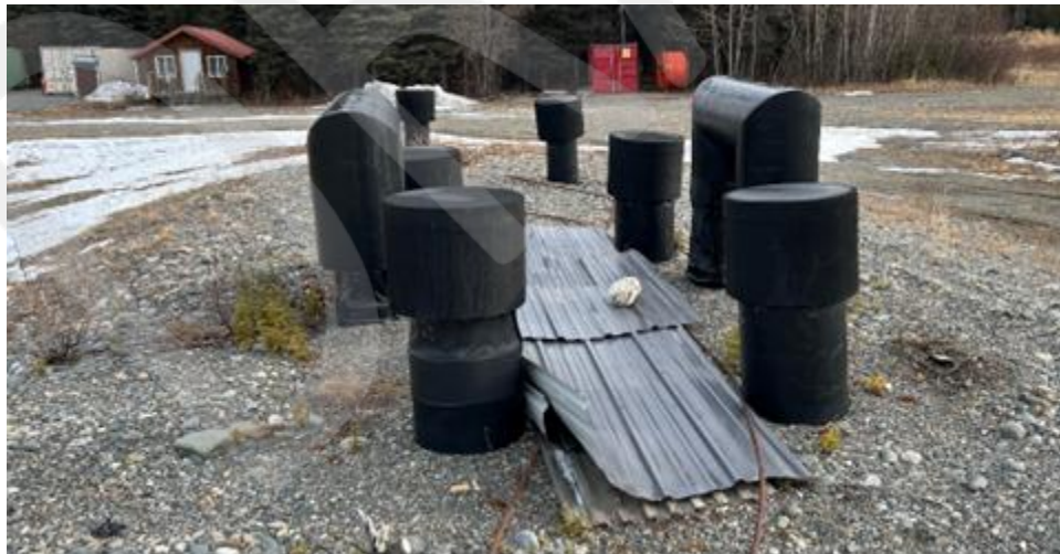
Figure 11. Community septic system for the Water Utility Building, Community Building and Tribal Office
