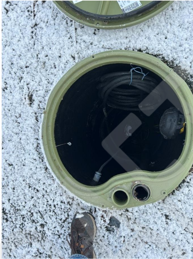
Figure 10. Lift station near Water Utility Building, with no evidence of insulation
