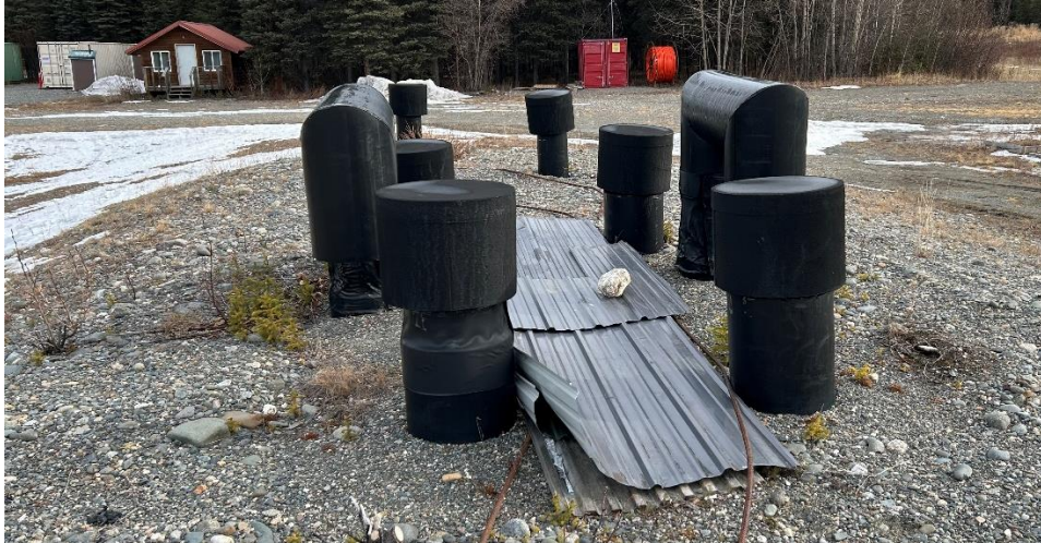
Figure 10. Community septic system for water facility building, community building and tribal office
