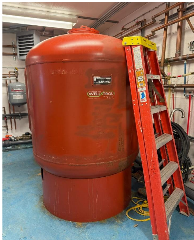
Figure 4. Pressure Tank in the Water facility Building
