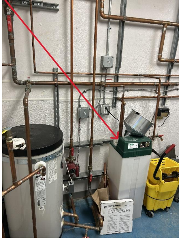
Figure 5. Cold water line to water heater. Red arrow indicates drain from cold water line into a glycol container, presenting a potential, but not immediately threatening cross-connection
