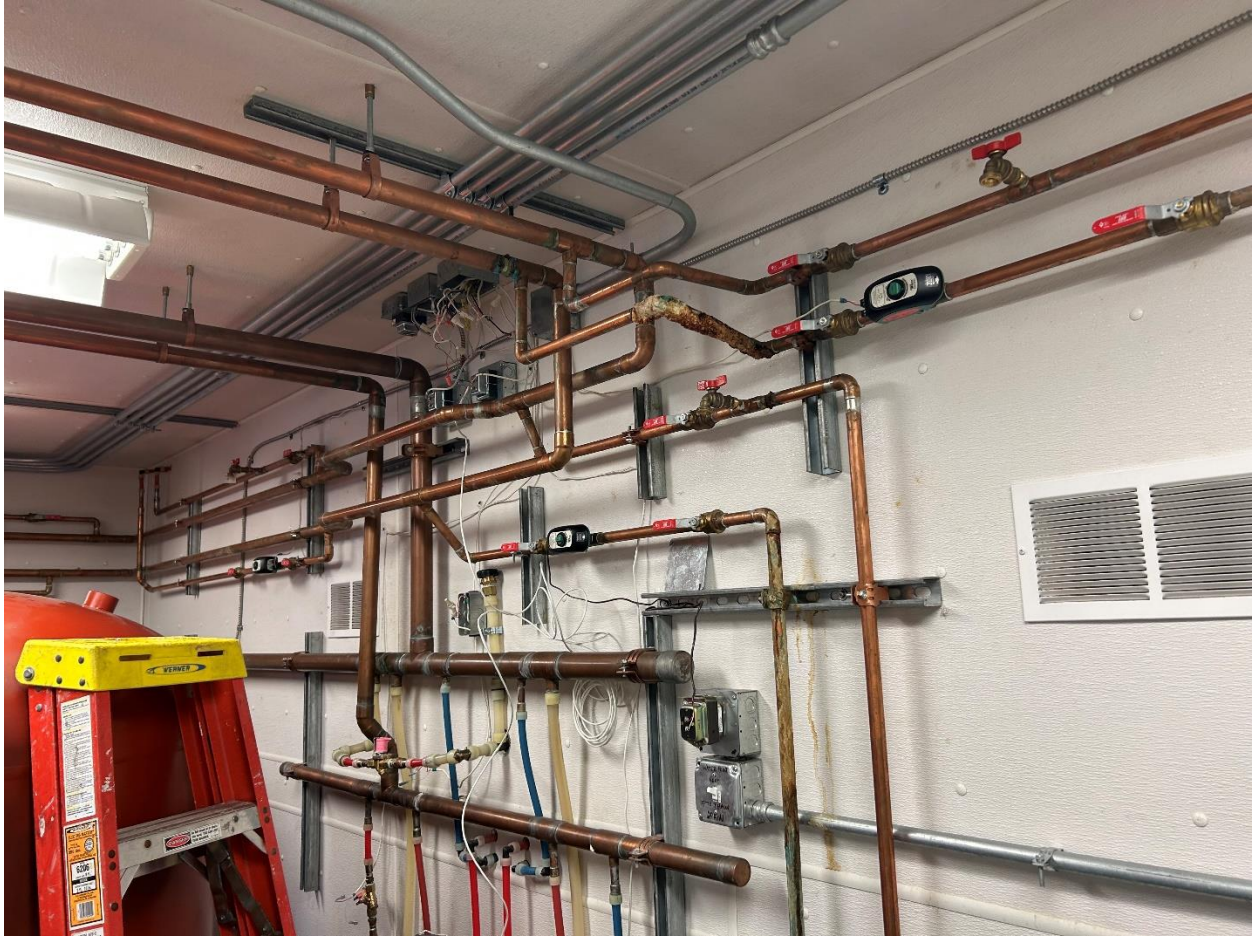
Figure 6. Pink valve in bottom left corner of this figure is the non-operational valve for the water fill point
