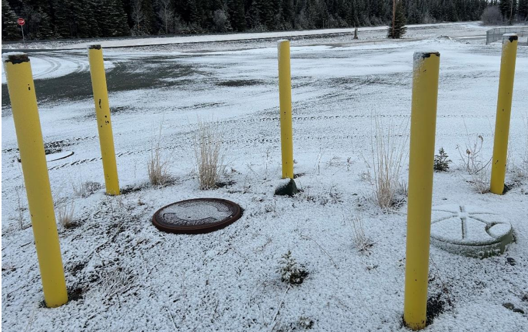
Figure 8. Lift station halfway between tribal office and water facility building
