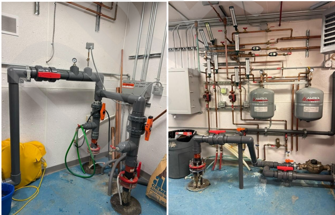
Figure 8. Water Utility Building's operation room
