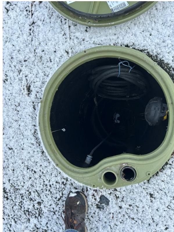
Figure 9. Lift station near water facility building, with no evidence of insulation
