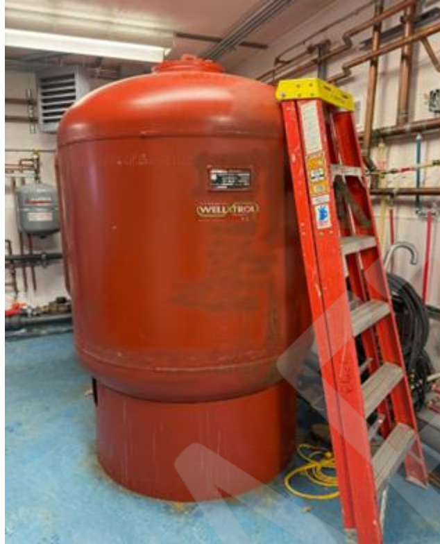
Figure 9. Pressure Tank in the Water Utility Building
